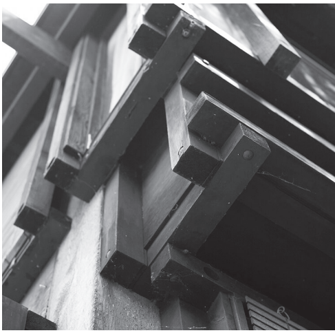
An interplay of timber and glass hung beyond the building enclosure, extends the width of the interior space.
