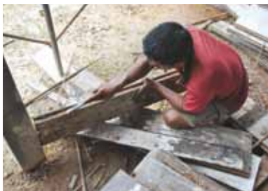
Old floor boards and wall panels were selected and processed for reuse.
