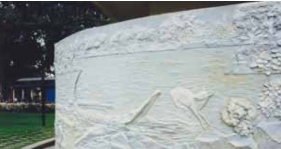
Concrete story wall - Designed by Conybeare Morrison and "carved" in concrete by Hasbee from Kalimantan. It depicts a popular Malay Folk tale about a mouse deer and a crocodile.
