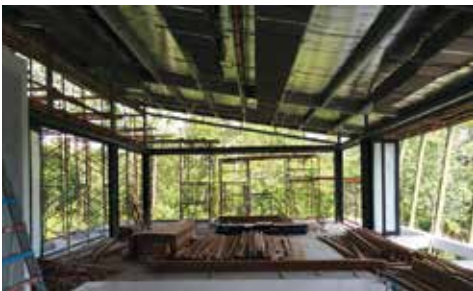
For the mono-pitch roof to work successfully it has to extend far enough from the face of building. (Rantau Panjang House by SML Architects.)
