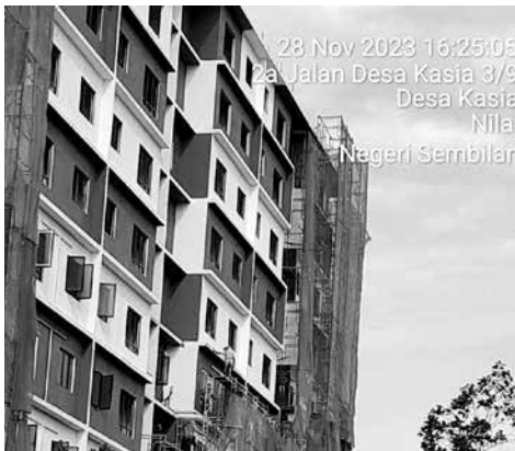
Meanwhile, via post COVID communication solution: site progress reporting via mobile devices is easy & satisfying, however it entails prompt response time from us too.
