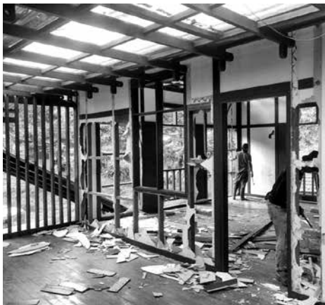
9.00am - The farm workers have started dismantling electrical appliances, GI conduits, window & door panels, toilet fittings to reuse and we sort out the timber based on sizes.
