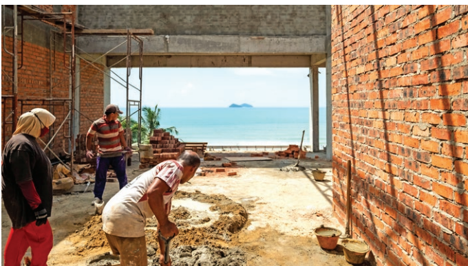
Construction of the apartment units with a view of Talang-Talang Island and the lapping waves of South China Sea.
