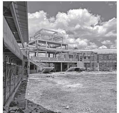
1:30am - site inspection of an upcoming school to check on progress and issues raised during the site meeting.
