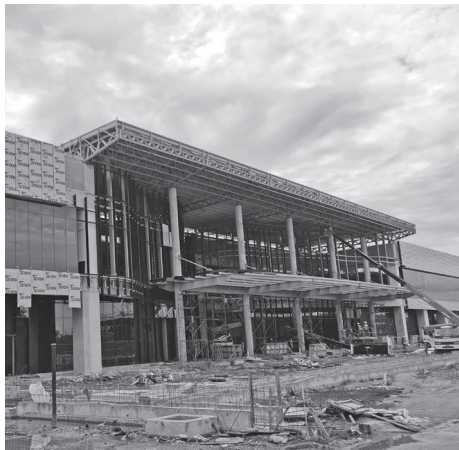
1.00pm - Inspection on the composite panel installation at a factory at Samajaya Industrial Park.
