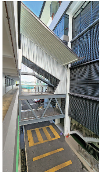
A new bridge that connects the existing classroom block with new admin block.
