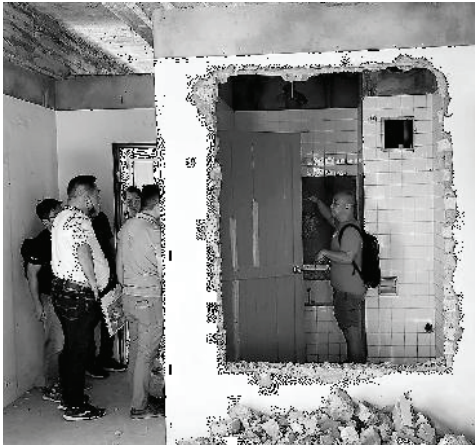
1.30 p.m. Hotel refurbishment project - site visit with sub contractors to finalise M&E routing.
