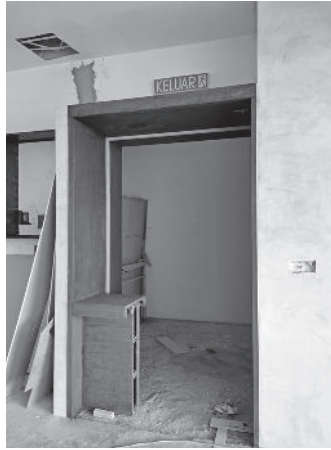
MAIN ENTRANCE - Oxidized metal door frame with delivery counter in position.
