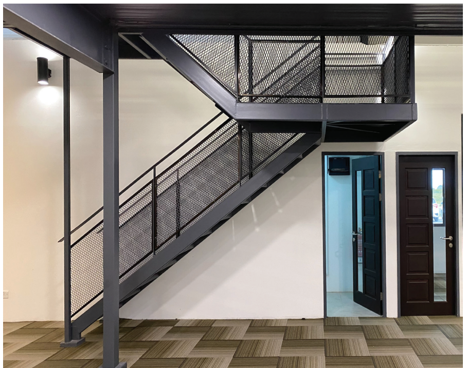
Steel staircase to the mezzanine floor office made of folded chequered plate threads and steel plate and expanded metal railings.
