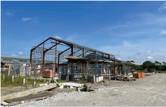
The main structure of the building consist of pre-fabricated mild steel for long span and fast construction.
