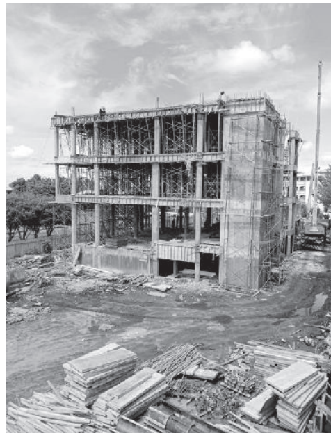
Construction was divided into 3 construction stages due to limited access into Site. The left wing and right wing of the building were only started after middle block was constructed.
