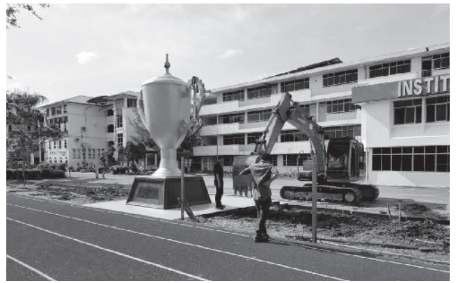
Protection works carried out for existing Trophy Statue and 100m Running Track.
