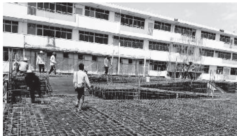
Construction of Upper Ground Floor Driveway Ramp, Drop-off Lobby (to connect the existing first floor classroom level).
