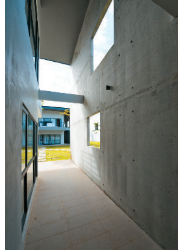
Openings on the off-form wall at corner units allows more natural ventilation and lighting.
