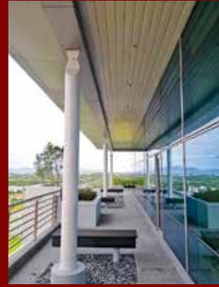
DML 100 G Aluminium Strip Ceiling - HSL Tower, Samarahan
