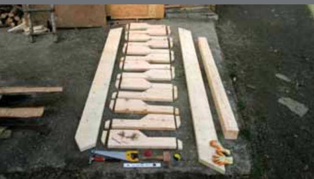
After completing the first staircase, we revised the existing design and built a space saver staircase; which took less time, materials and manpower. This is probably the first space saver staircase in Romania.
