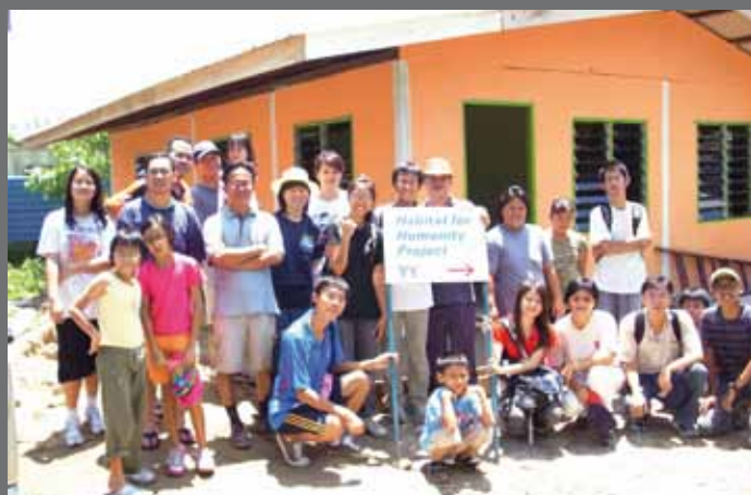
Weekend build - volunteer of all ages get to work with the Home-owners
