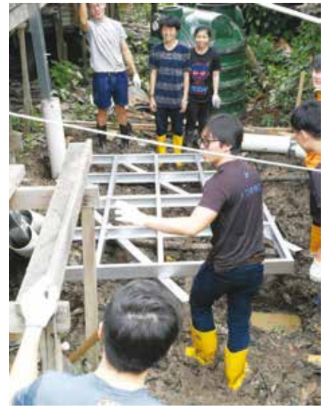
The floor structure being prepared for final connection to the steel columns.
